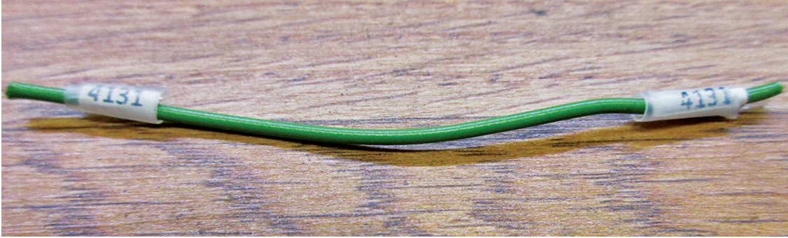
Labels on the ends of a wire with shrink-sleeving over them. Even for very short wires, it is highly recommended to put labels at both ends.
