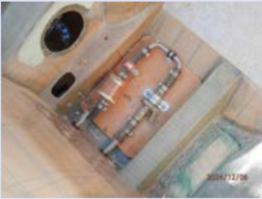
Fuel Filters - Installed
